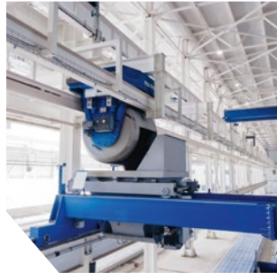
Concrete distribution system
